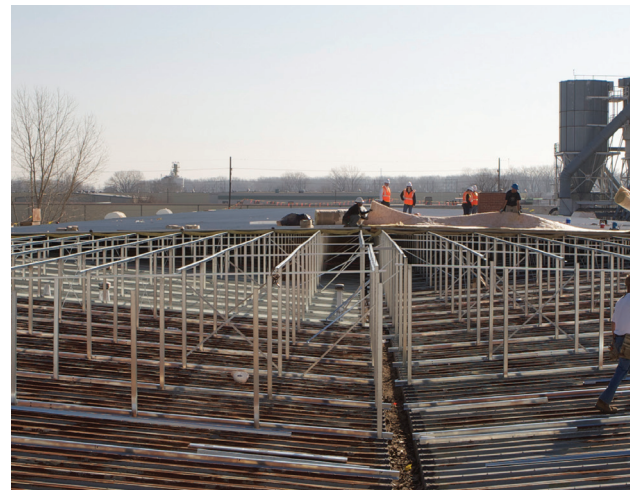
A Butler reroofing system is a long-term solution that saves the cost and inconvenience of tearing off an existing roof.
